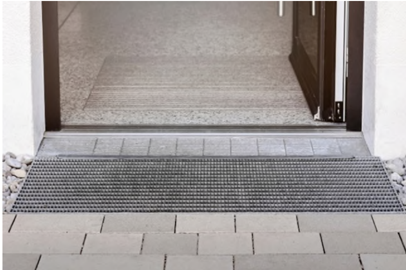
Figure 4.6 Channel drain at entrance door
