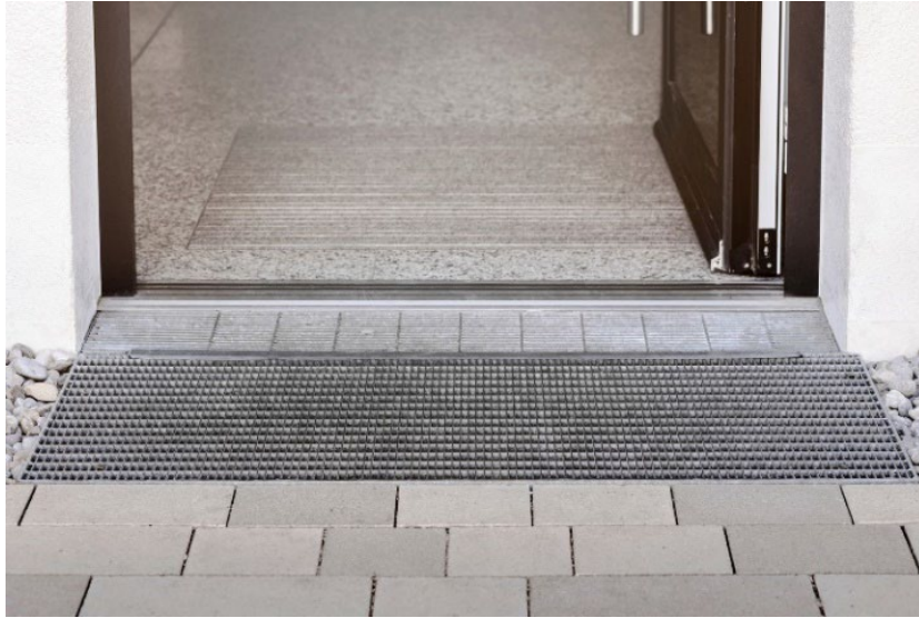
Figure 4.6 Channel drain at entrance door
